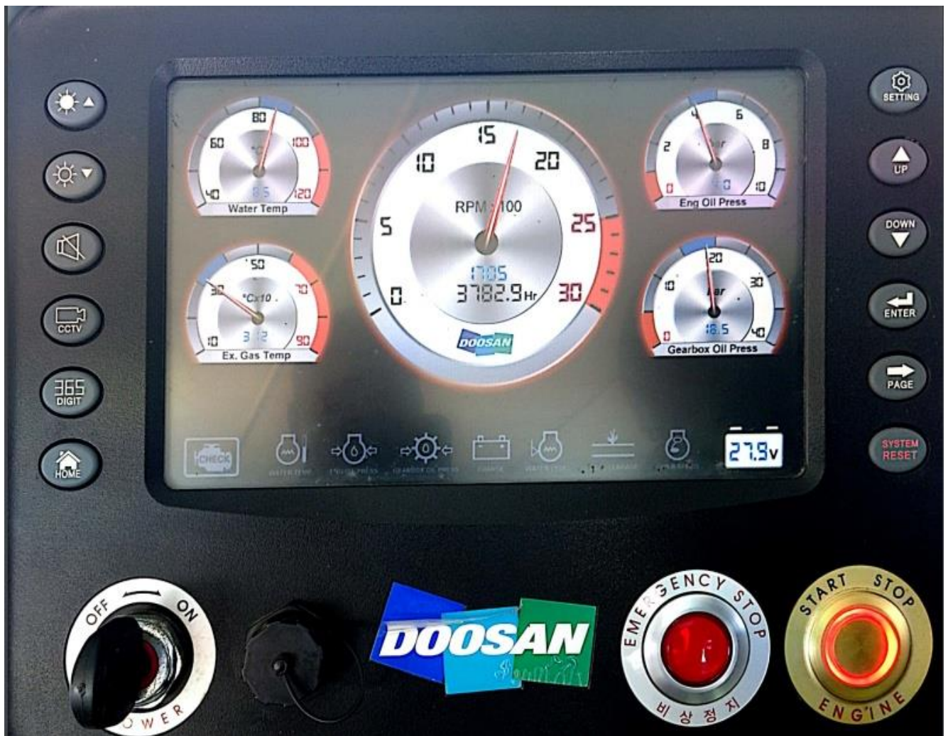
Figure 5.0: Mv Kazi dash board for RPM and Engine running Hours Parameters, Doosan Engine Control and Monitoring Panel" or "Doosan Engine Management System."
